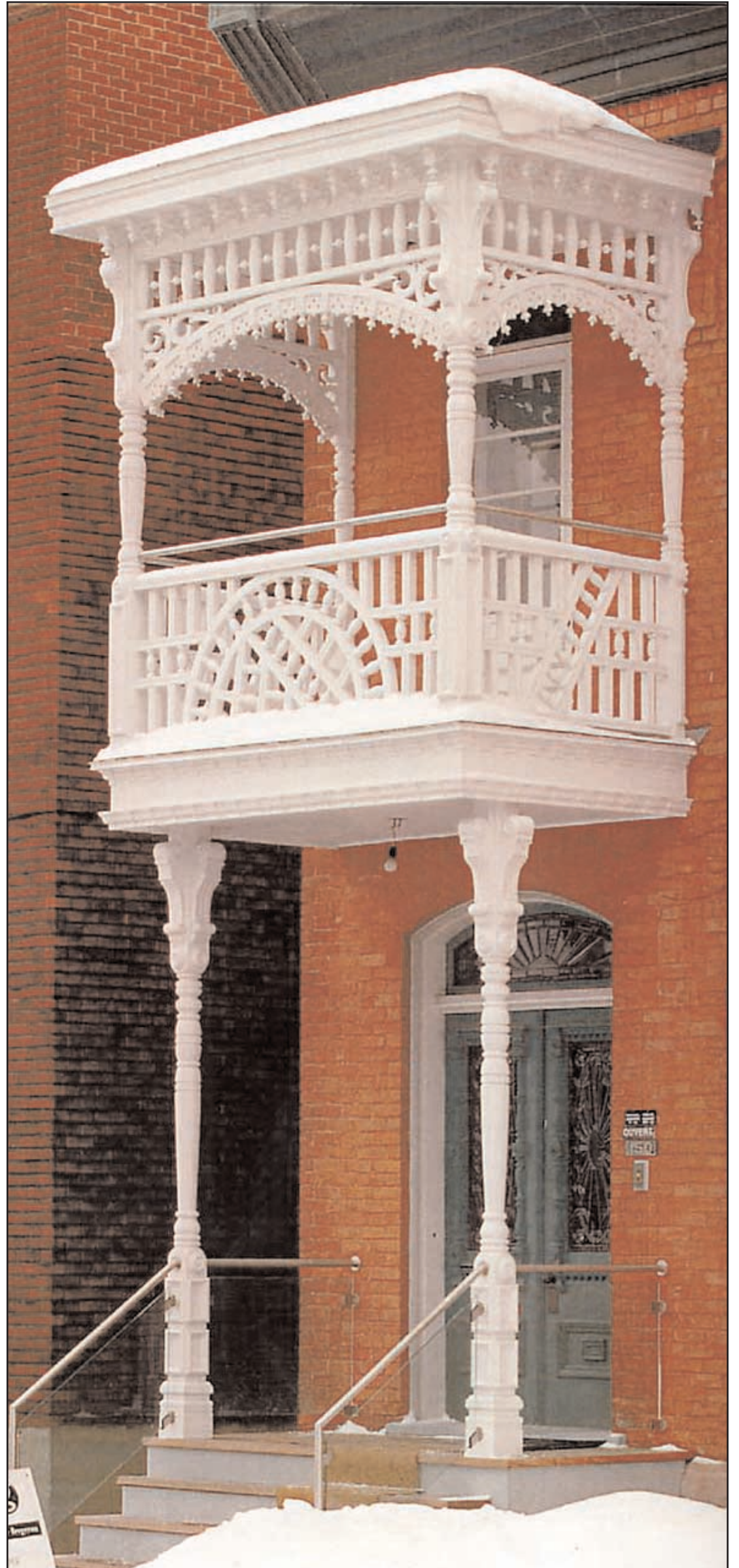
The restored porch at 150 St. Patrick is as intricate as the long vanished original and captures its glory.
